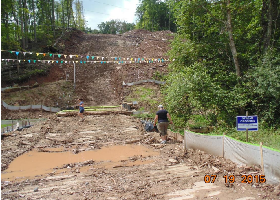
Stream crossing at Stonewall Gathering Pipeline construction site on Copley Rd., about 2 miles west of I-79 in central Lewis County, WV
