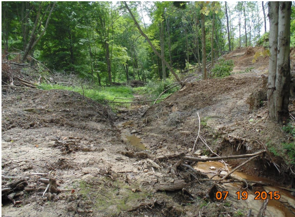
Stream crossing at Stonewall Gathering Pipeline construction site on Elk Lick Rd., 6.25 miles west of I-79 in northern Lewis County, WV
